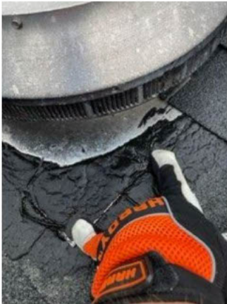
areas around the base of a roof vent where tar is deteriorating and allowing for possible water penetration.
