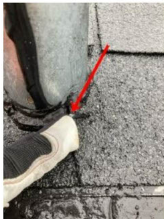
hole observed where previous patch job has failed around the base of a vent
