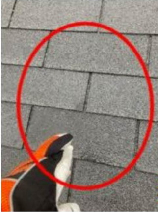
area along front right of home where roof is spongy
