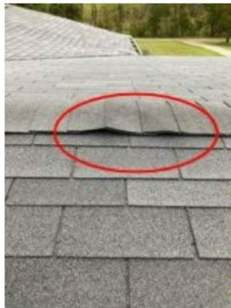
ridge cap shingles are lifting and allowing for possible water penetration
