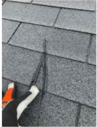
what appears to be sliced shingles that were poorly patched with tar
