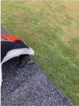
damaged shingle along the rake edge
