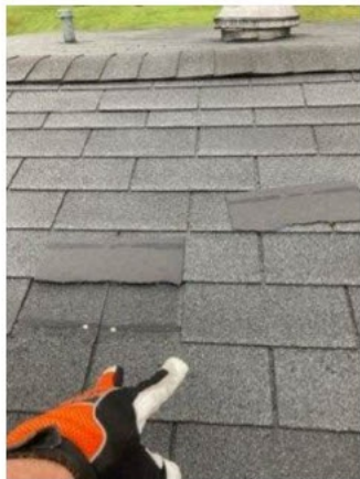
missing shingles and exposed nails
