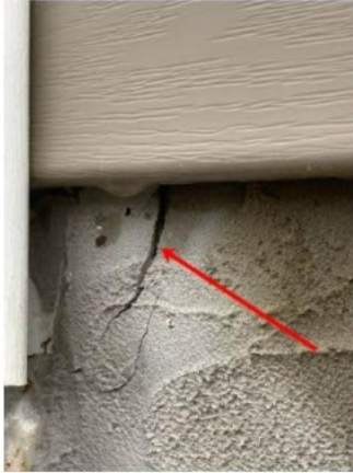
crack observed near the left front corner of the home. No evidence of flashing was observed between the siding and foundation.
