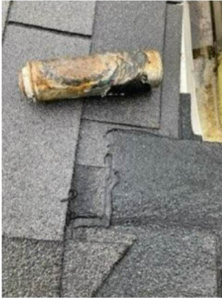
more tar at the base of the roof and an aerosol can found in the gutter
