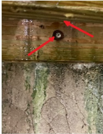
Flashing missing under deck ledger and rusty lag screw washer indicating regular moisture
