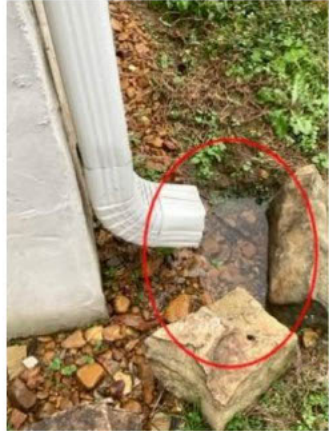
water pooling at the foundation from gutter discharge during a rain event.
