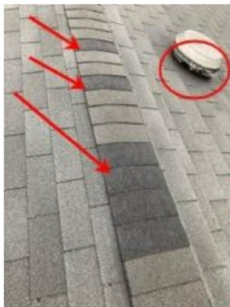
evidence of prior repairs to roof cap shingles. Also damage to roof vent can be seen in the background.
