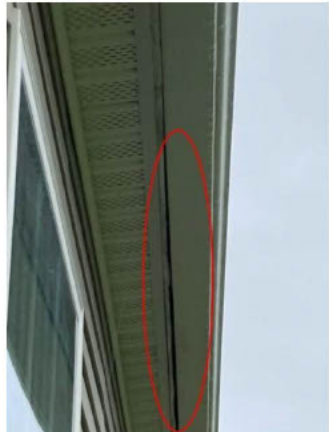
guttering was observed pulling away from the fascia board at the rear of the house. The homeowner indicated that it had also occurred and been repaired at the front of the home.
