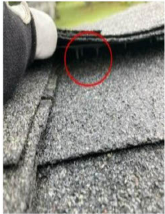
Nails showing where ridge cap shingles are lifting
