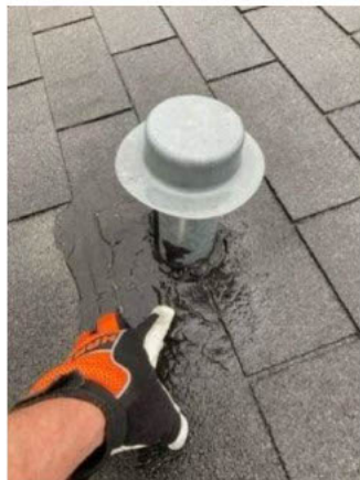
tar repair around vent penetration
