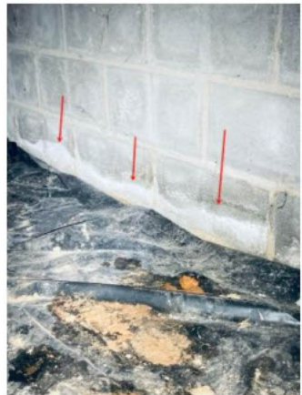
Efflorescence observed at the base of the foundation where water at the exterior of the home (under the ramp at the front of the house) appears to be accumulating from a combination of loose guttering, poor drainage around the foundation, and lack of flashing between the siding and the ledger board.
