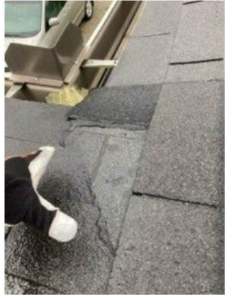
poor patch job at the base of the valley where water enters the gutter. Kickout/diverter flashing appears to be properly installed.
