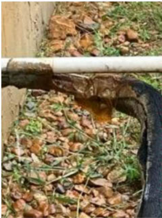
Insulation is damage and missing on the suction (return) line of the condenser unit. Recommend new insulation be installed
