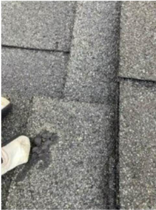
previously tarred and improperly installed nail that is again becoming exposed
