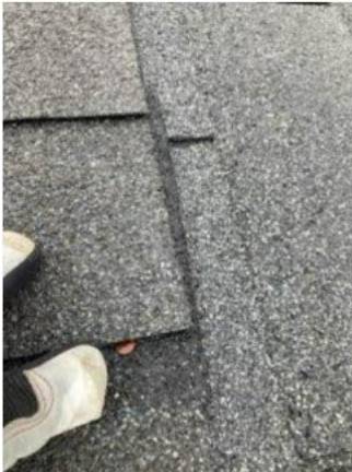
exposed nail head just showing below the overlapping shingle
