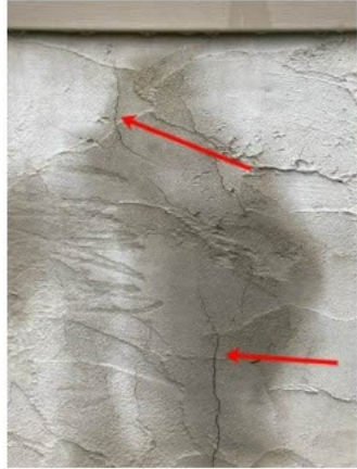
cracks observed in stucco treatment on the foundation where possible moisture intrusion is occurring
