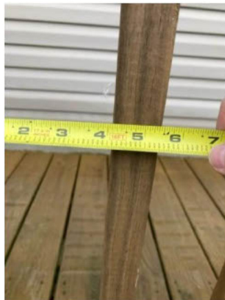
railing spacing should not allow a 4" sphere to pass.
