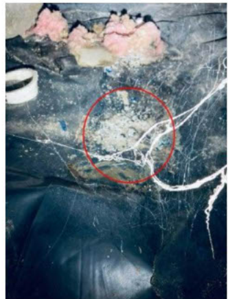
small area where waste water has accumulated from a slow leak in the pipe.
