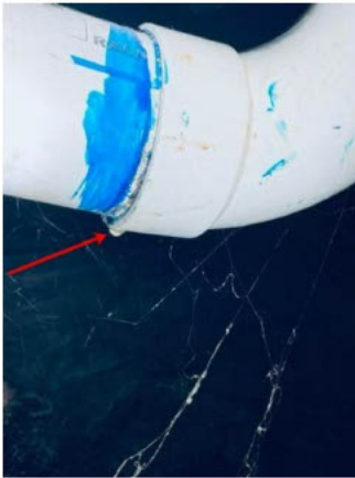
slow drip observed on a drain pipe under the crawlspace at the right rear of the home.
