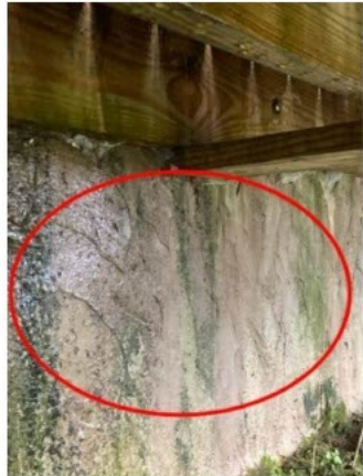
Algae growth under the front deck ramp indicating moisture accumulation
