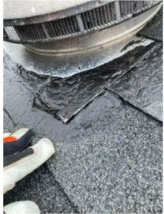
tar deterioration around the flashing of a roof vent
