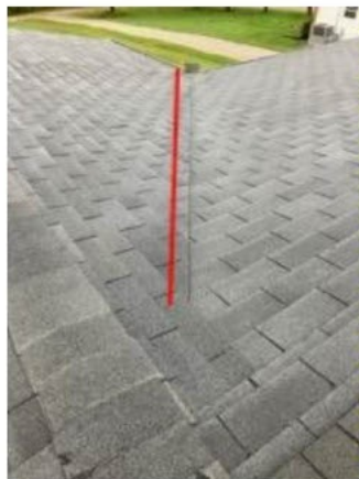
closed cut valley improperly installed with shingles cut along valley center. Should be offset 2" to the lesser drainage side as red line indicates.
