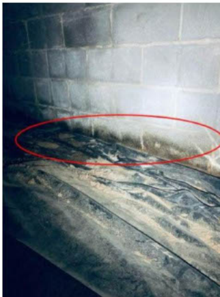
mold-like substance observed under the crawlspace at the foundation wall where water appears to be accumulating at the exterior front of the house (under the deck).
